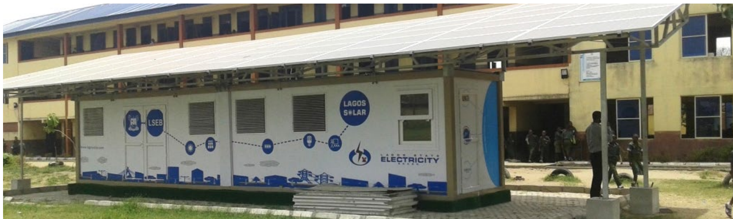
Full exterior view of solar and storage solution for schools and PHC's throughout Lagos State, Nigeria
