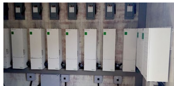
Installation consisting of MPPT 80 600 charge controllers and XW+ inverterchargers
